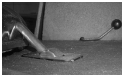
Fig 3 - Flue damper open
